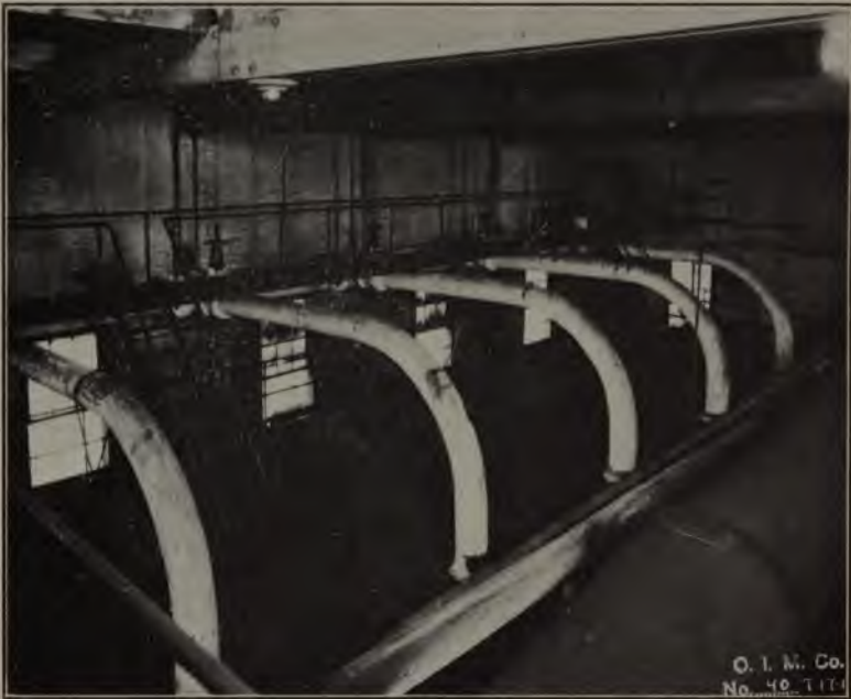
No. 7—Spruce Mine, Top of Boiler Setting, Eveleth, Minn.
